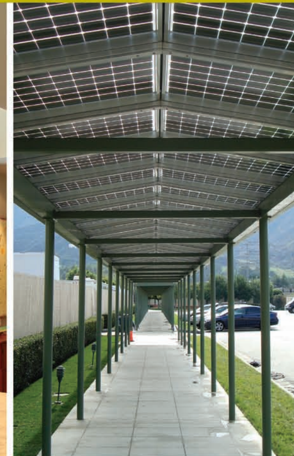
Breezeway: 44kW El Solutions Burbank, CA
