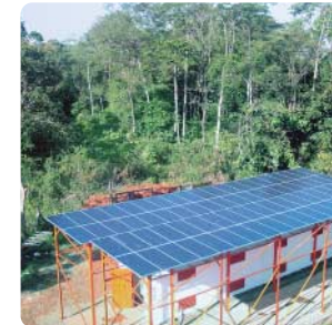
Remote telecom base station
