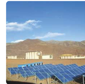
Small power plant
