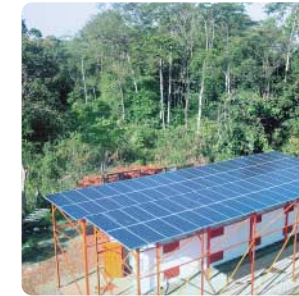
Remote telecom base station
