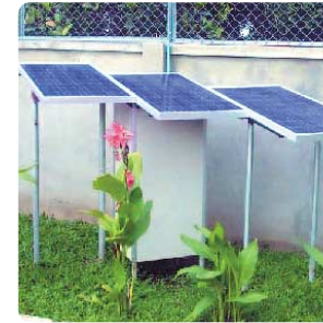
Solar home system
