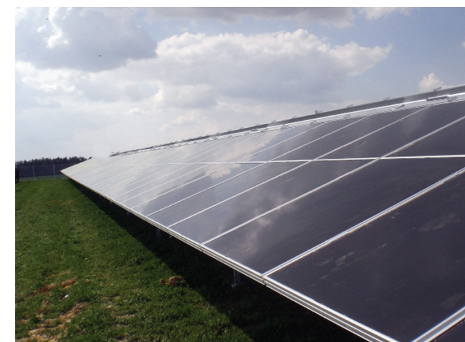
Sharp thin film products offer high performance for multi-megawatt power generation.
